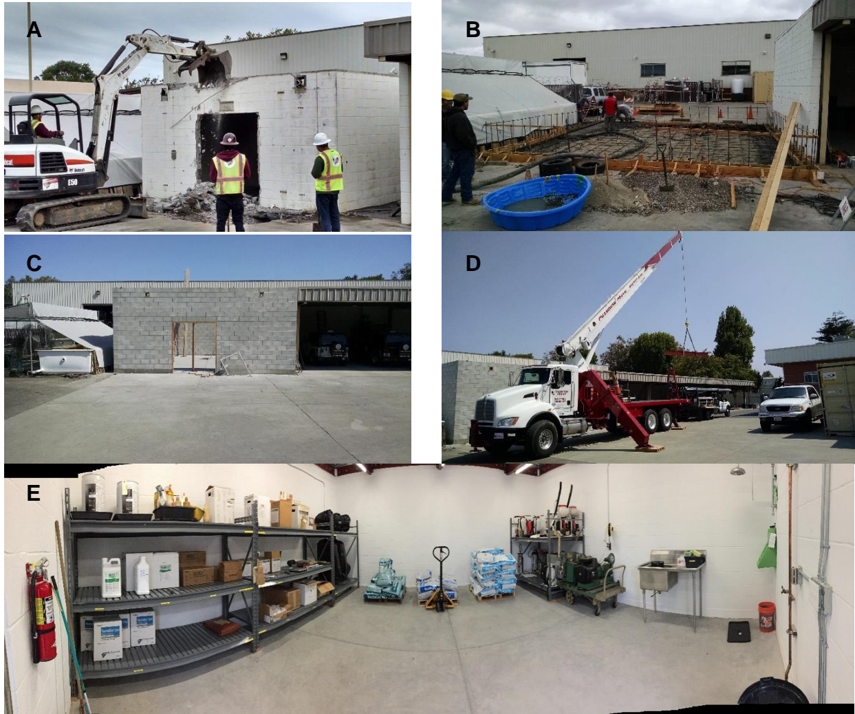
Figure 26. Pesticide storage shed remodel project. (A) Demolition of the old pesticide storage shed. (B) Construction of the foundation for the new larger pesticide storage shed. (C) Completion of the foundation and walls for the new shed. (D) Hoisting the steel beams for the roof of the new shed. (E) Interior view of the completed pesticide shed.
