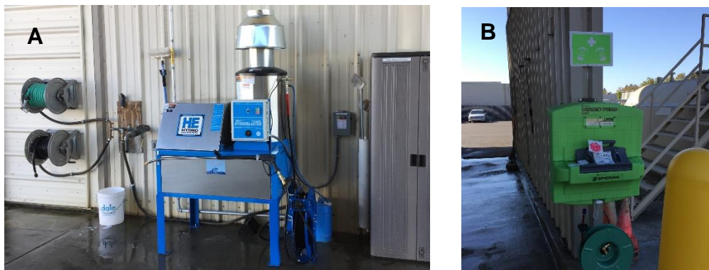
Figure 28. Wash rack improvements. (A) New pressure washer system. (B) New eye wash station.
